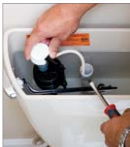
Check your toilet for leaks.
