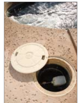
Pool fill valve
