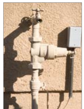
House gate valve
