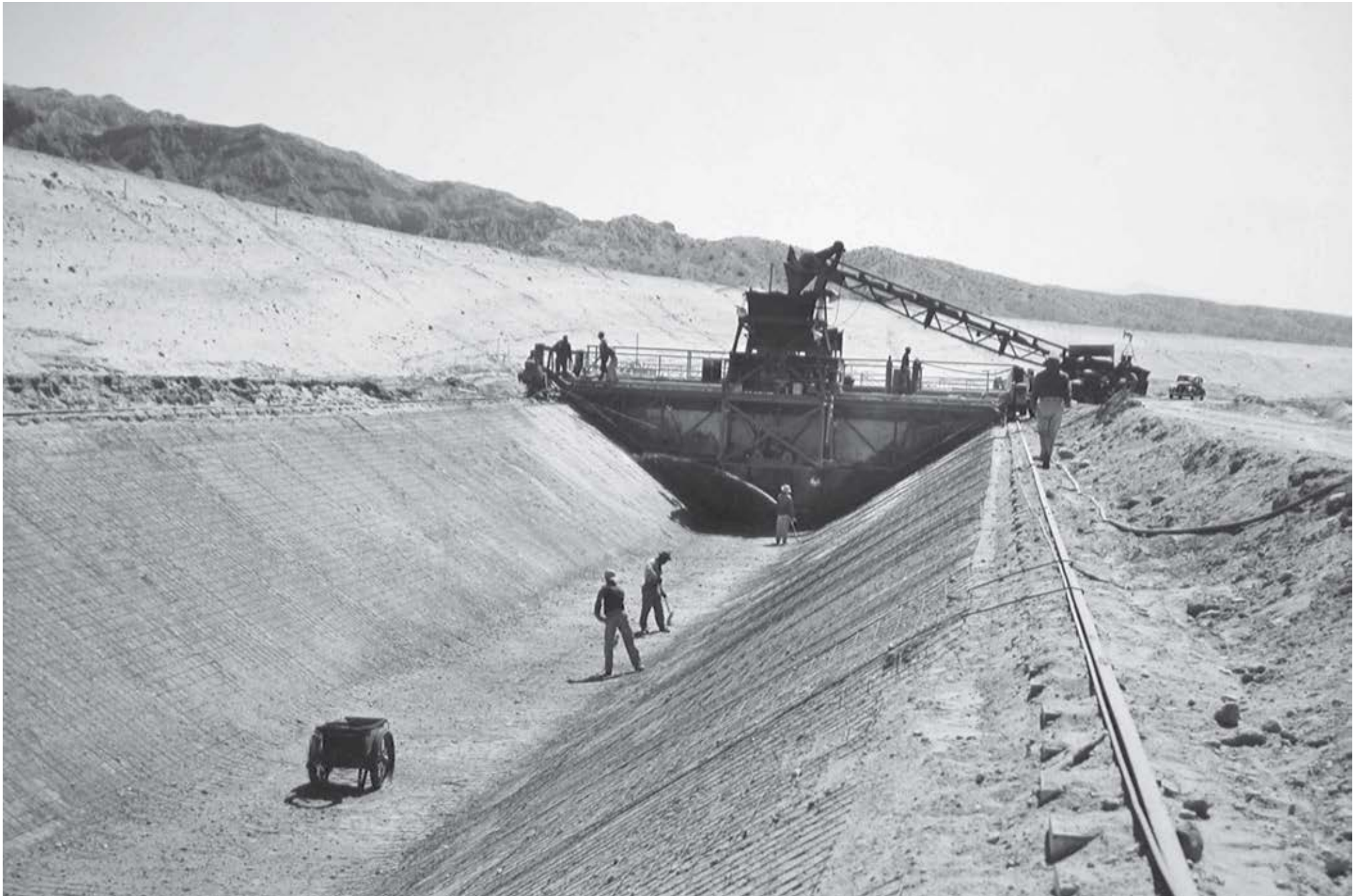
Workers start to place concrete on the service area of the Coachella Branch of the All-American Canal. CVWD archive photo
