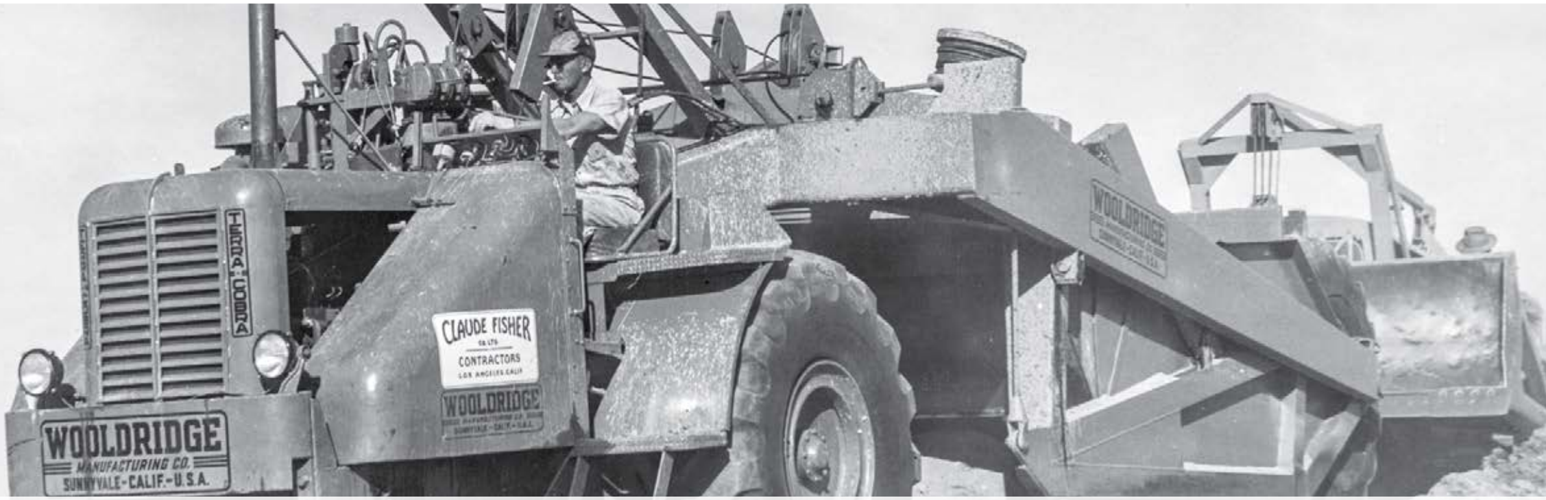
Heavy equipment was used for much of the All-American Canal construction. CVWD archive photo
