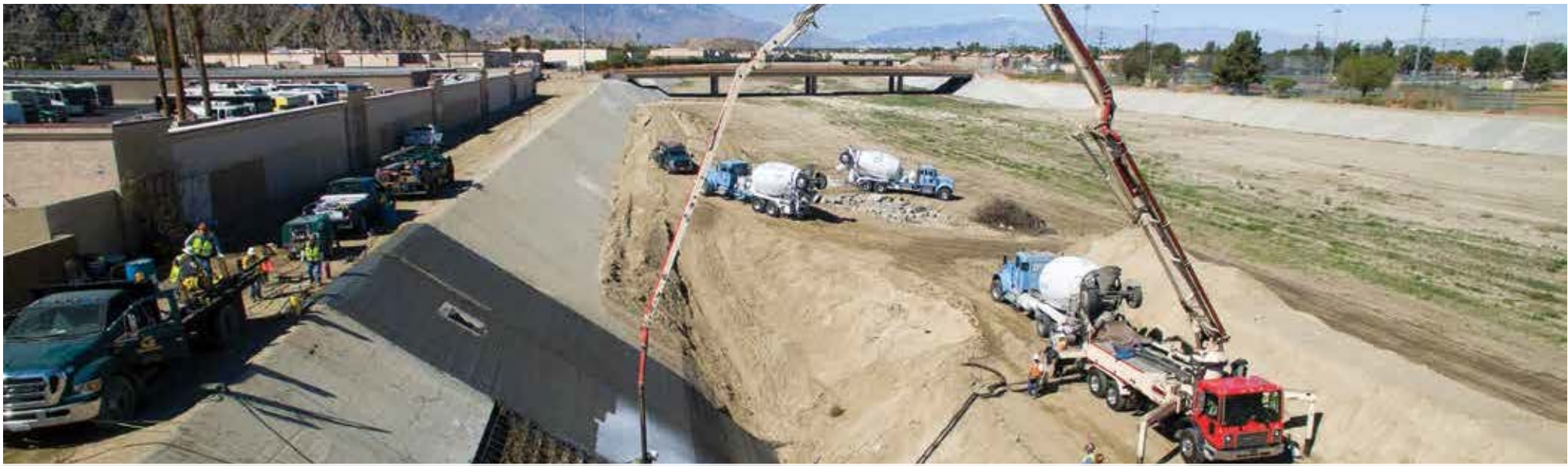
A crane with a boom is needed for repair work along the Whitewater River Channel after a storm. CVWD archive photo
