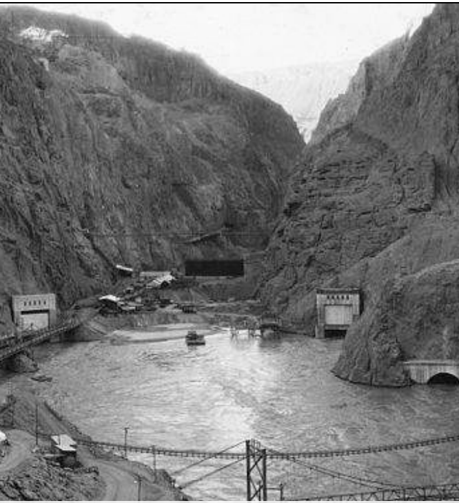
Construction workers had to create diversion tunnels to redirect the Colorado River while they were building Hoover Dam. This photo was taken in 1933. Courtesy of the U.S. Bureau of Reclamation
