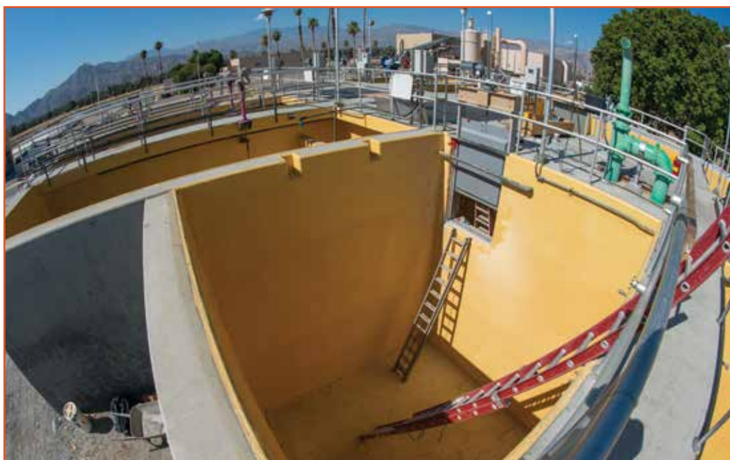
Tertiary Filter Improvement Project at WRP 10
