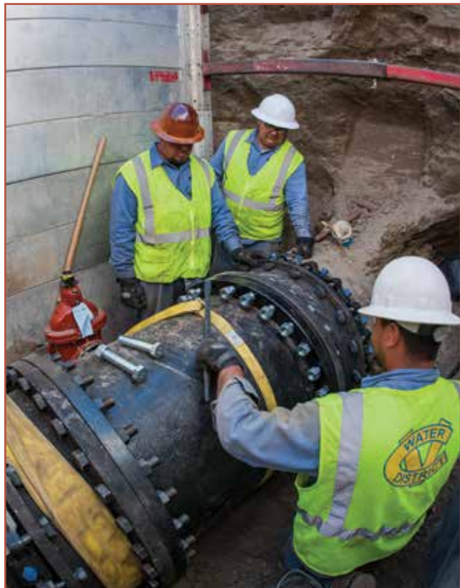
Crews cut a section of a water main and replace it with a distribution manifold that had two 12” butterfly valves.
