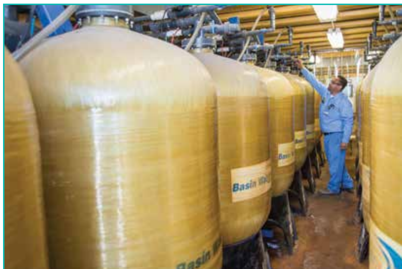
CVWD's Ion Exchange Plant in Mecca, CA
