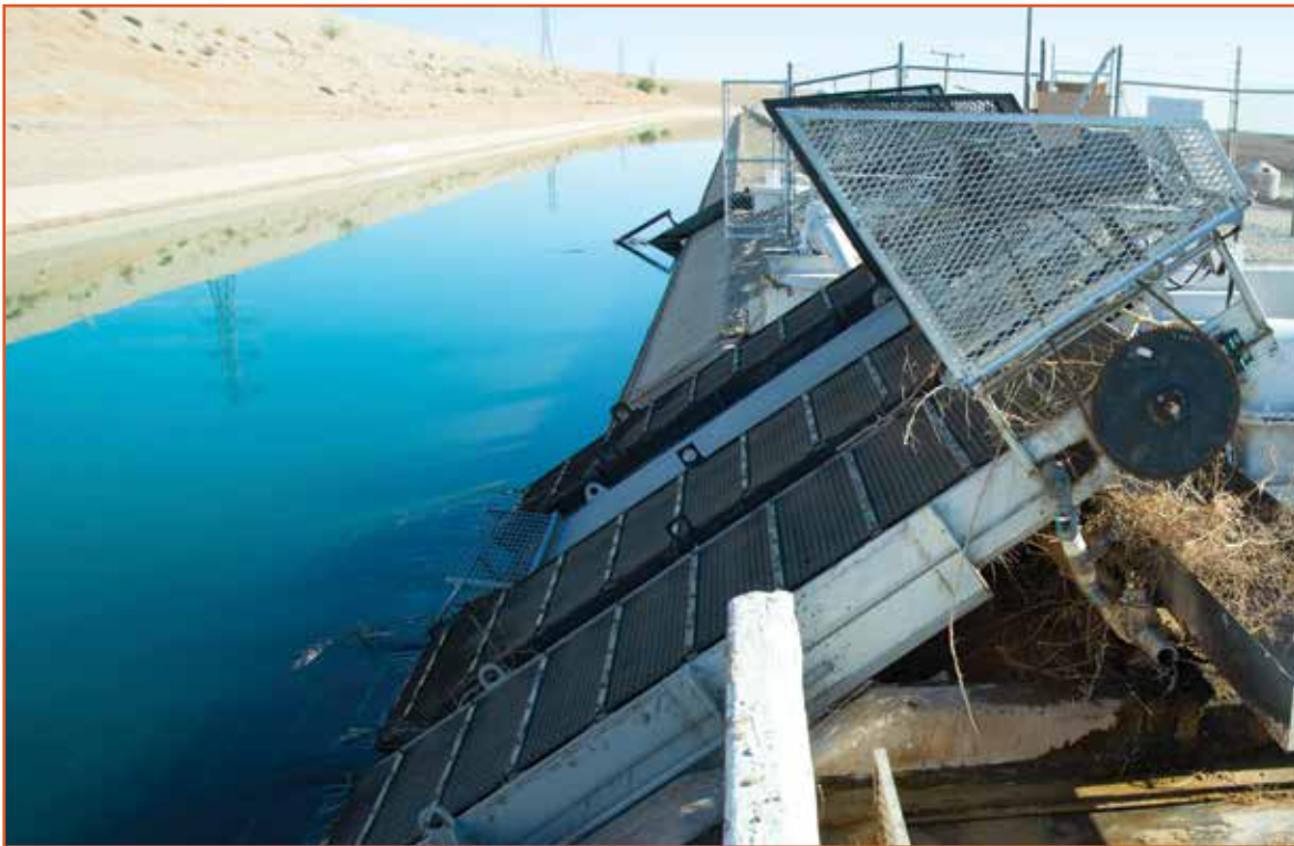
Traveling screens removing debris on the Coachella Canal
