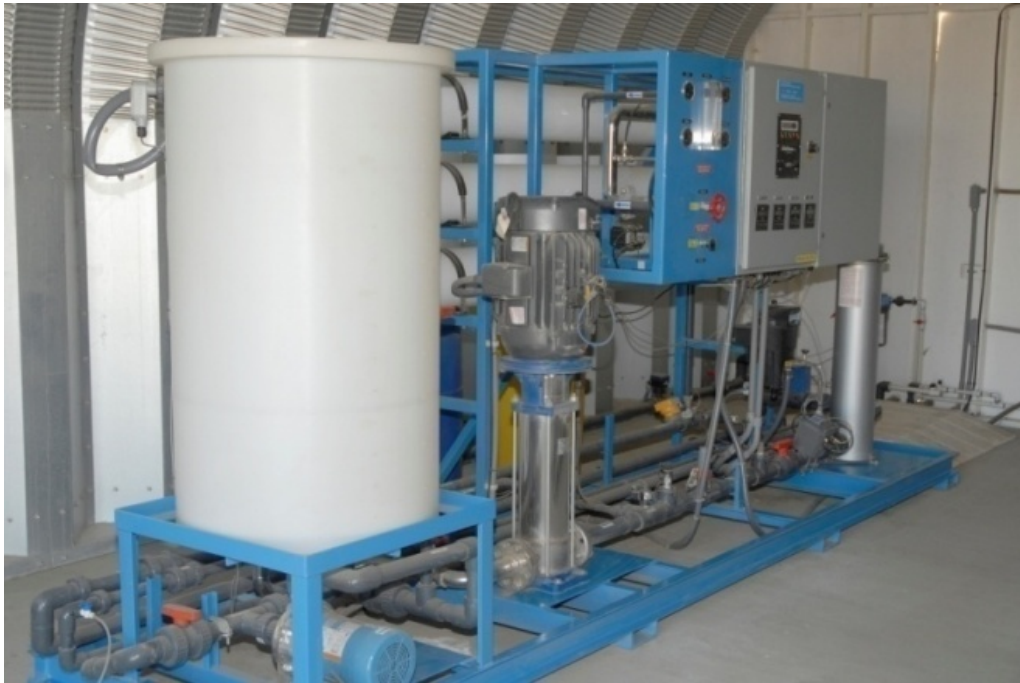
Figure 4-4 Drain Water Desalination Pilot Facility
